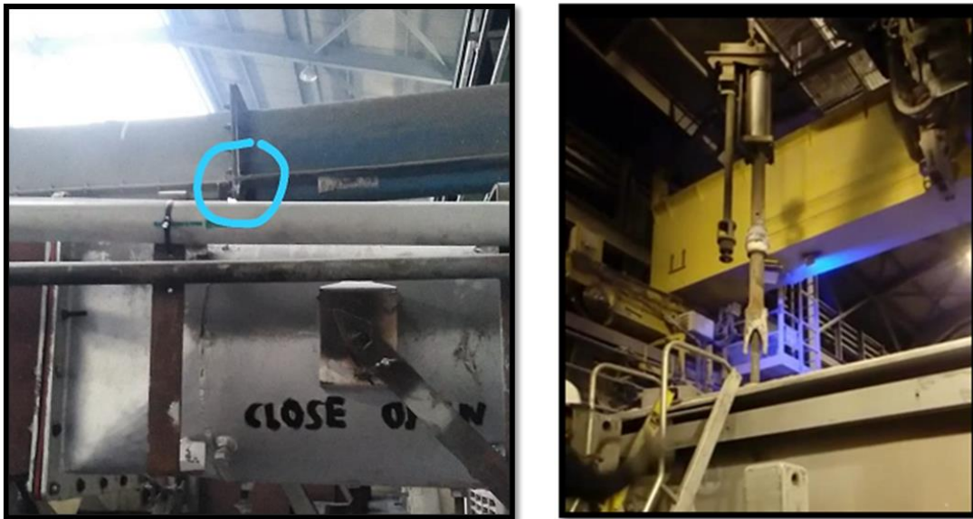
Figure 4. Air slide connection (left) and CAFD placement (right).
