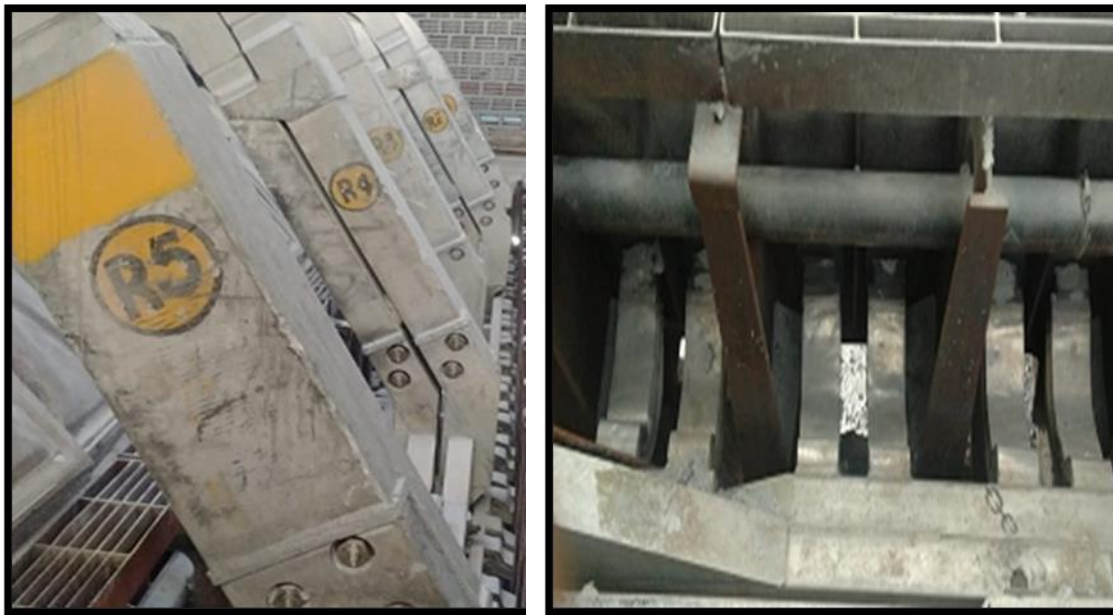
Figure 3. Anode risers (left) and cathode clads (right) can be worked in parallel.
